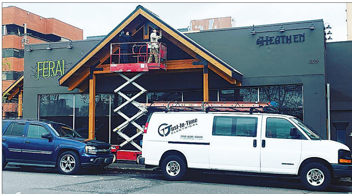
Courtesy of Just-In-Time Electrical
